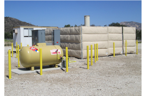
Groundwater system equipment, covered by sound blanket
